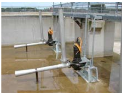
Guide rail mounted in oxidation ditch
