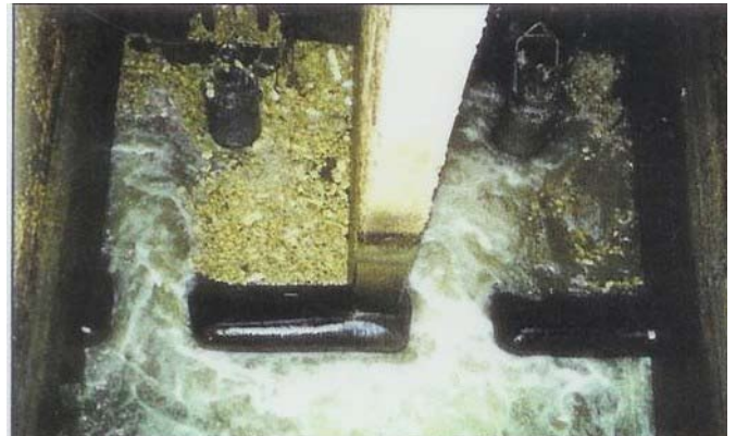
Floating material is entrained and pumped from the wet-well
