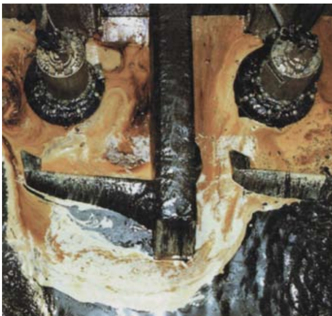
Skimming floating oil from sump
