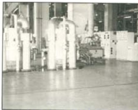
Process plant flooring Fabrieksvloerbedekking
